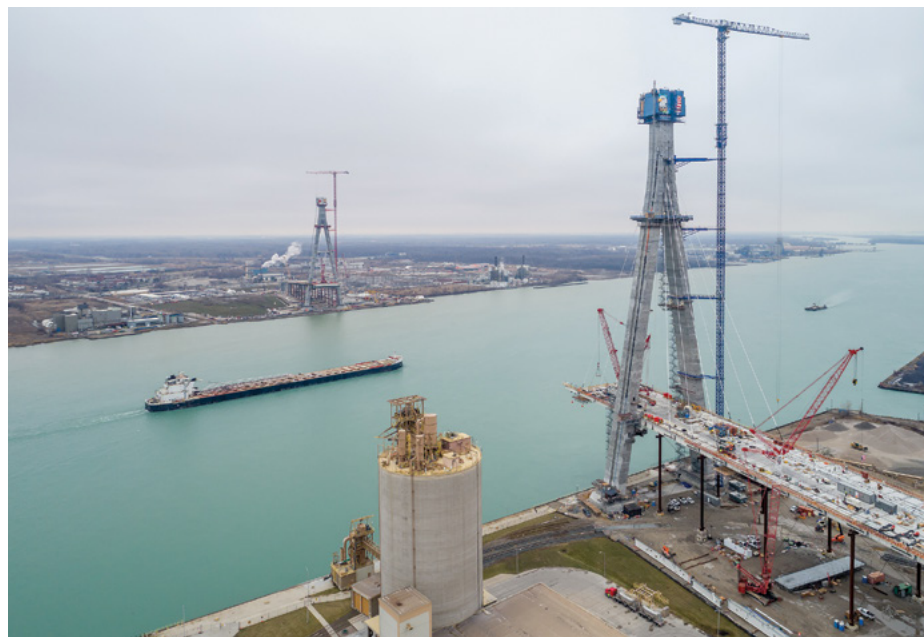
Freighter passing along the Detroit River in between the Bridge Pylons and road deck extensions. Photo by Pat Brennan.
