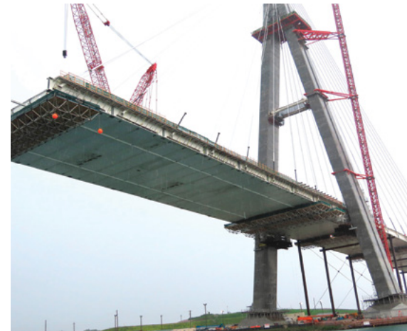
Gordie Howe International Bridge Pylon and road deck extension. Photo by Pat Brennan.
